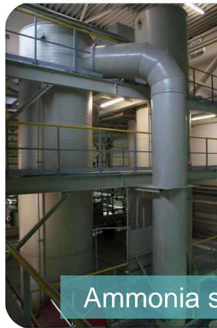
Pump & heat exchanger room
